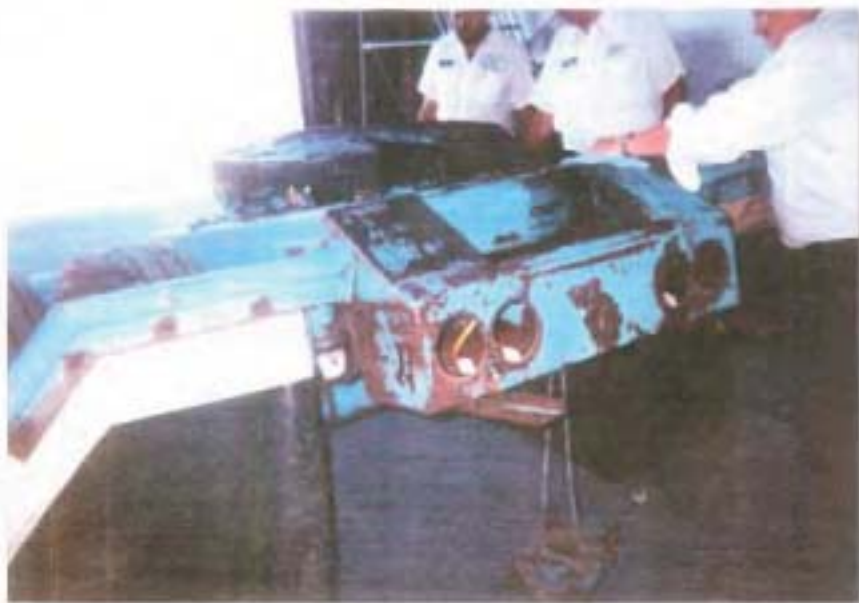
TRUCK DOLLY BEFORE APPLICATION OF RUST GRIP. DOLLY WAS POWER WASHED ONLY IN PREPARATION FOR COATING.
