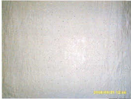
<EnamoGrip coated area>
